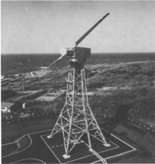
Fig. 7. A 100 kW wind power generation pilot plant.
