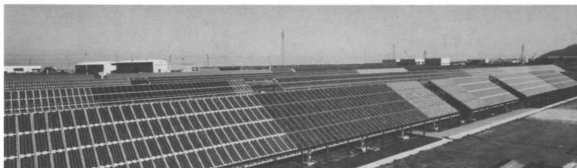
Fig. 4. A 1 MW photovoltaic central power station.
